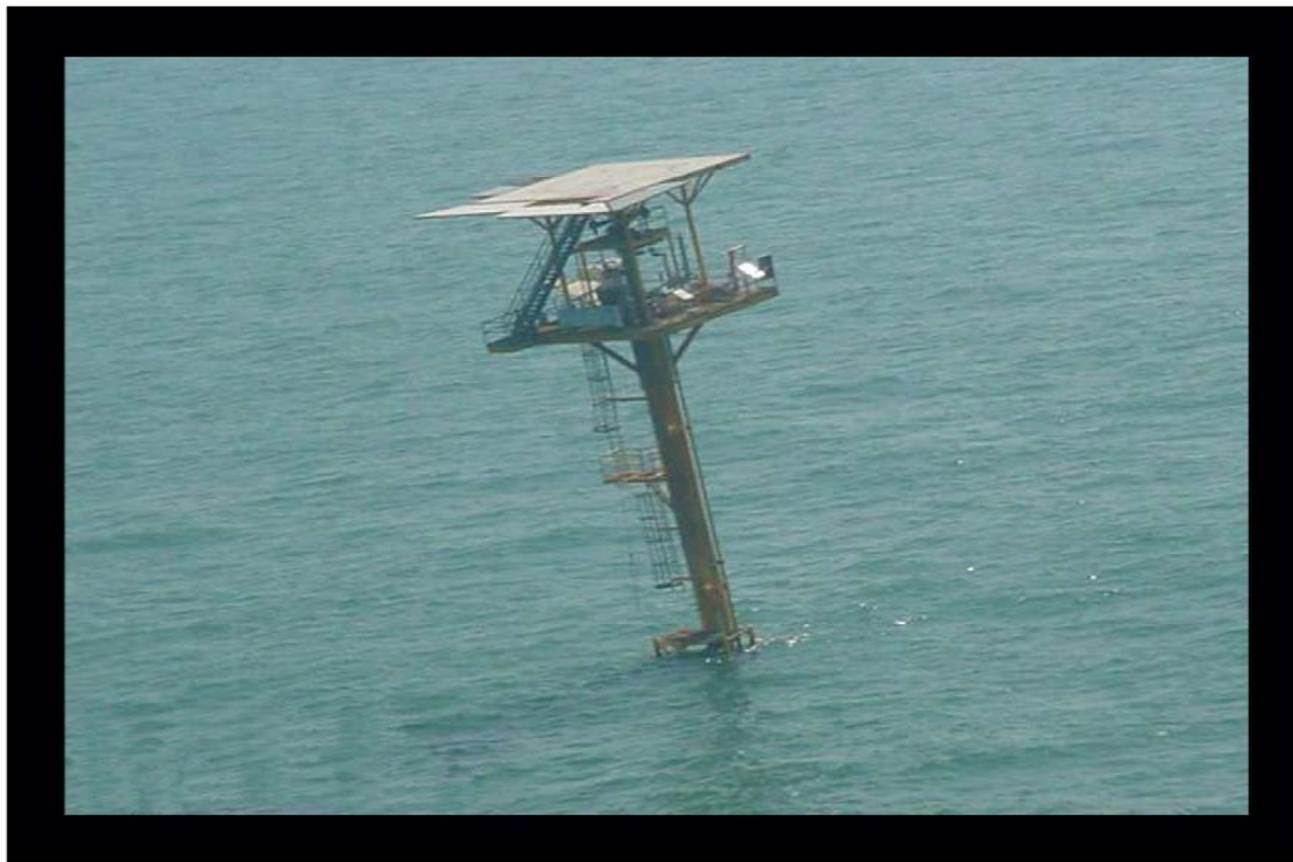
Damaged Single-Well Caisson: The vast majority of damage occurred to small, older platforms. Damage ranged from stripping of decking and rails to bending of well jacket and in some cases total removal of all above sea level structural components.
